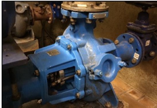
Sludge recirculation pump.
